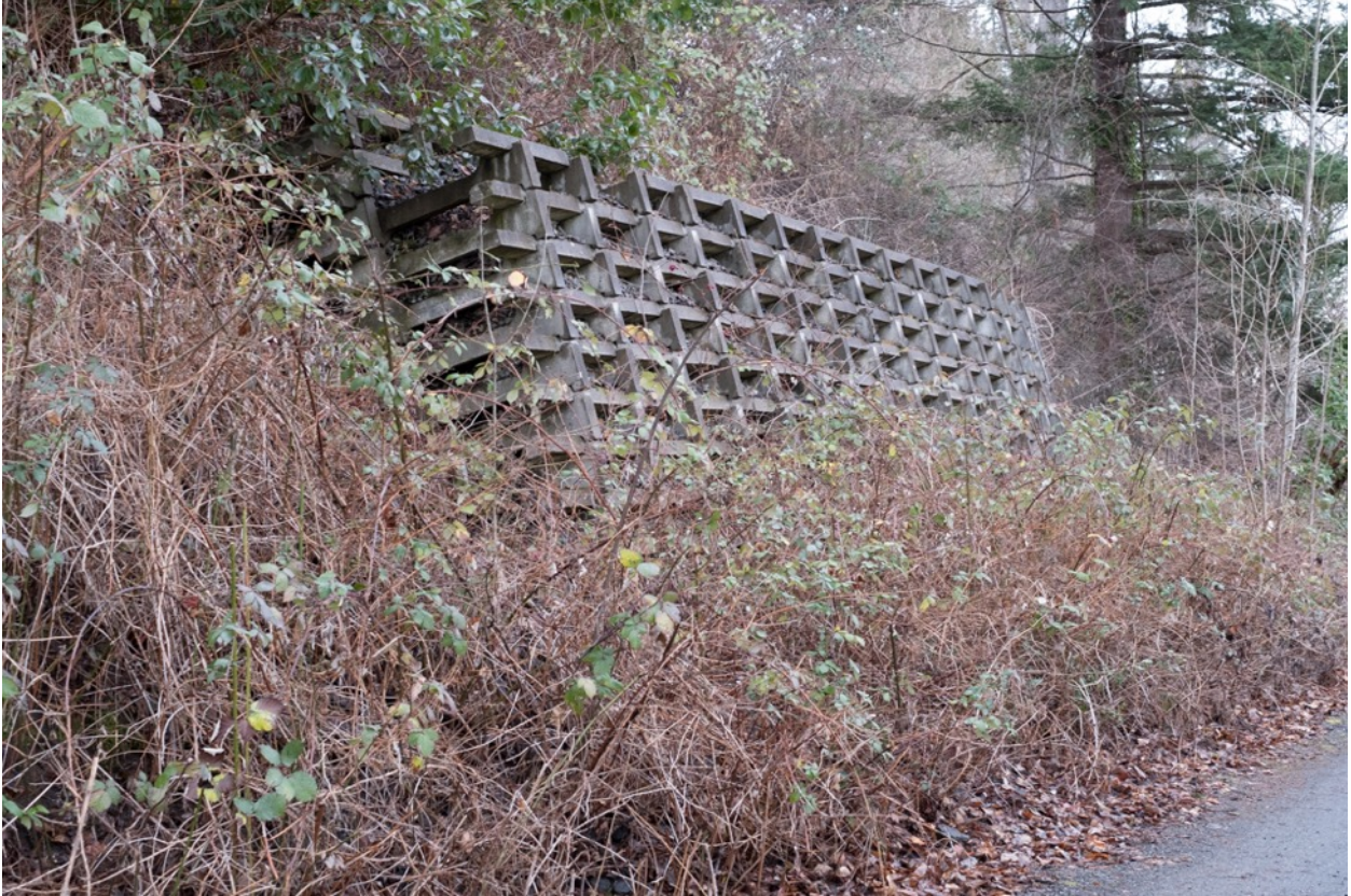
Retaining Wall supporting house and property from collapsing during rains. This must be protected or our property will be at risk from a landslide – which also endangers the trail itself.
