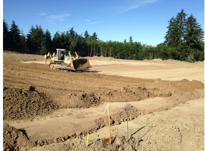
Above: Preparing the subgrade for the building pad. They are placing lifts of native soil, rolling and testing.
